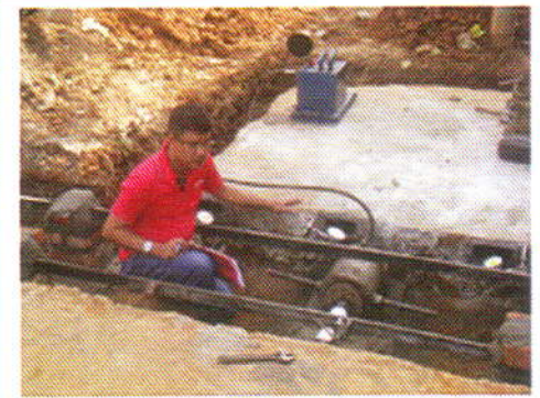
Performing Full Scale Pile Cap Lateral Resistance at Civil Engg. Dept., Assam Engg. College (OIL-IEI, ASC H P Barua Fellowship-2014)
