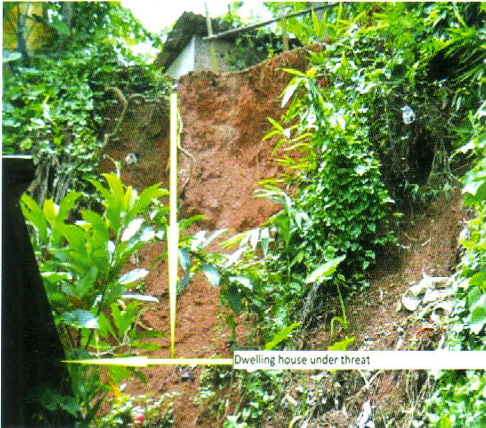
Fig-1: A Man Made Slope in Refinery Colony Area
